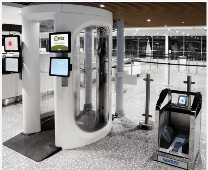
Passenger Screening by Combined System (WTMD and SECURITY SCANNER) and Shoe Scanner (SAMDEX)
